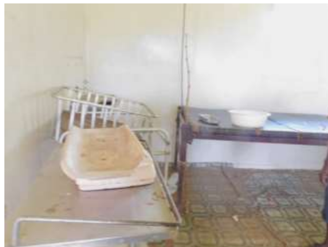
The dilapidated labour ward at Aiome Health Centre
